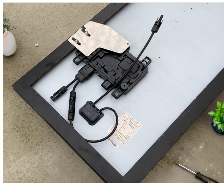
Figure 7: The fixed microinverter on the back of the Solar Deck
