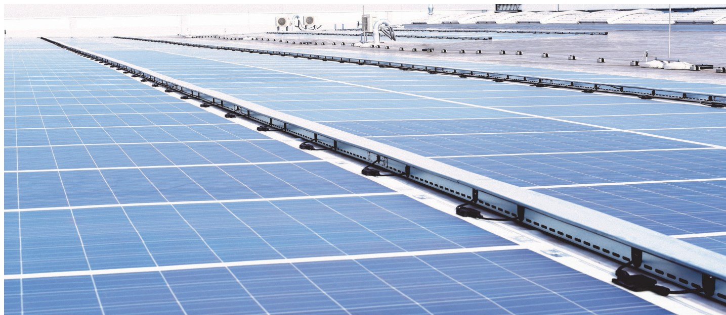
Rooftop installation DAS Energy Headquarters
