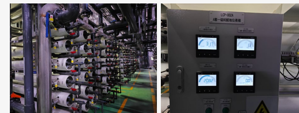
Primary RO Equipment and Local Instrument Box at the Pure Water Station
