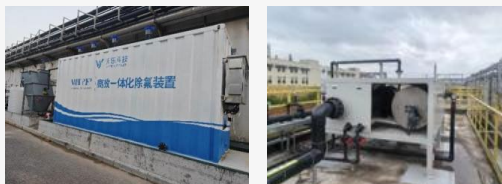
Calcium Fluoride Sludge Defluoridation Unit
