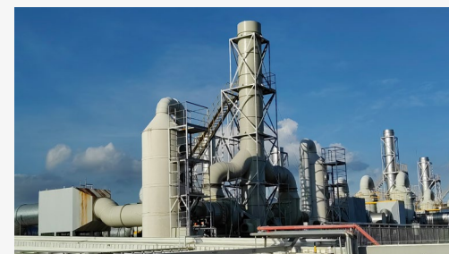
Organic Waste Gas Treatment System Installed at Module Thermal Exhaust Outlet
