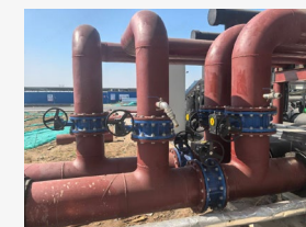
Chiller System Free Cooling Project Equipment
