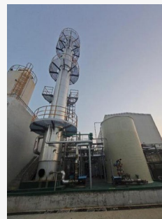
Ammonia Water Recovery Facility
